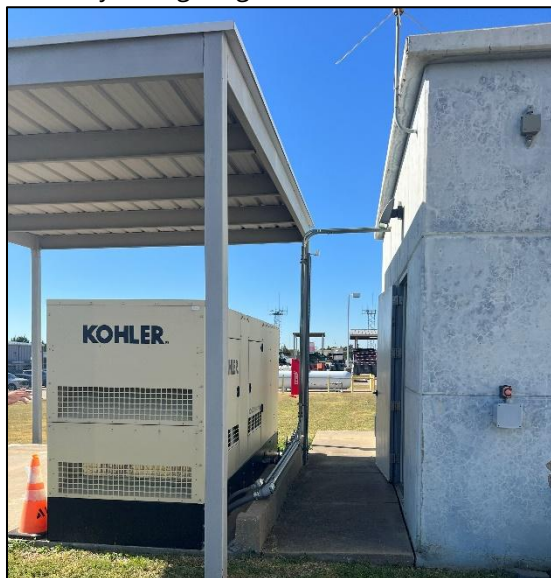
Airfield Lighting Vault and Generator
